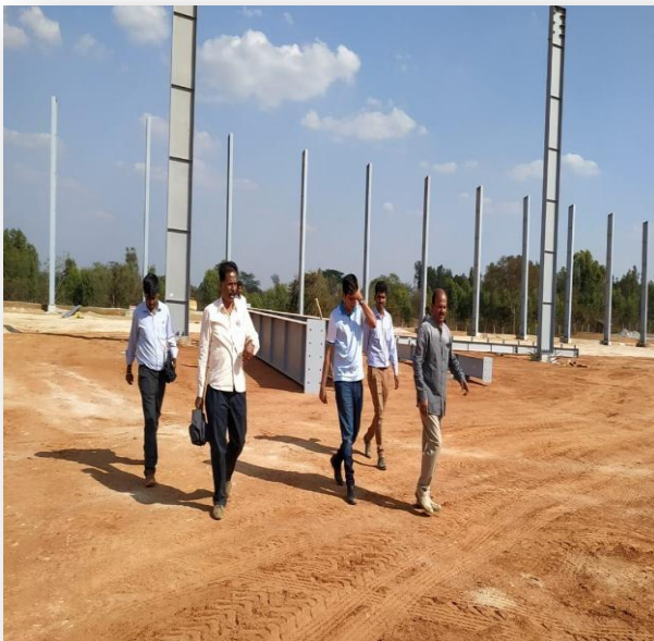
Site visit by our faculty Sri C S Vijaykumar for inspection of Pre-Engineered Buildings
